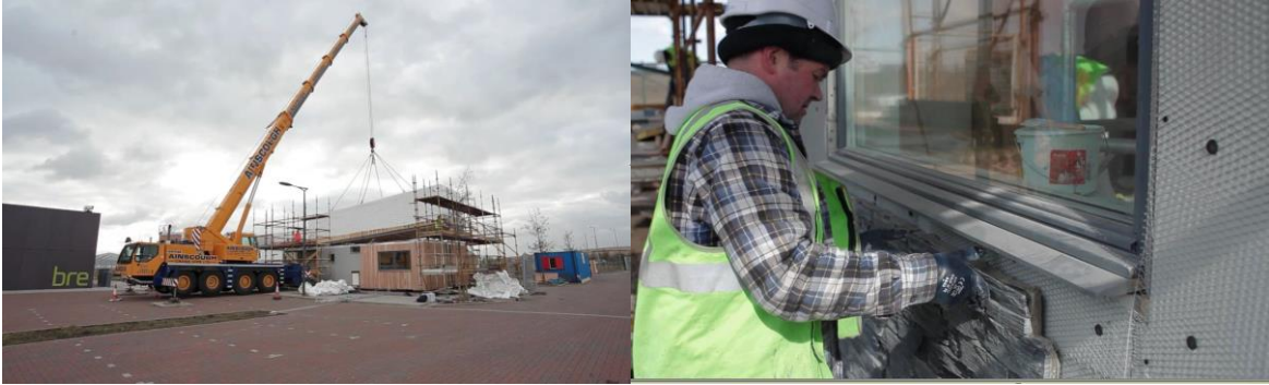
“The stone cladding panels were applied on site – as they would have been too heavy to transport safely. The stone on the panels is recycled.” Gary Bennett.
