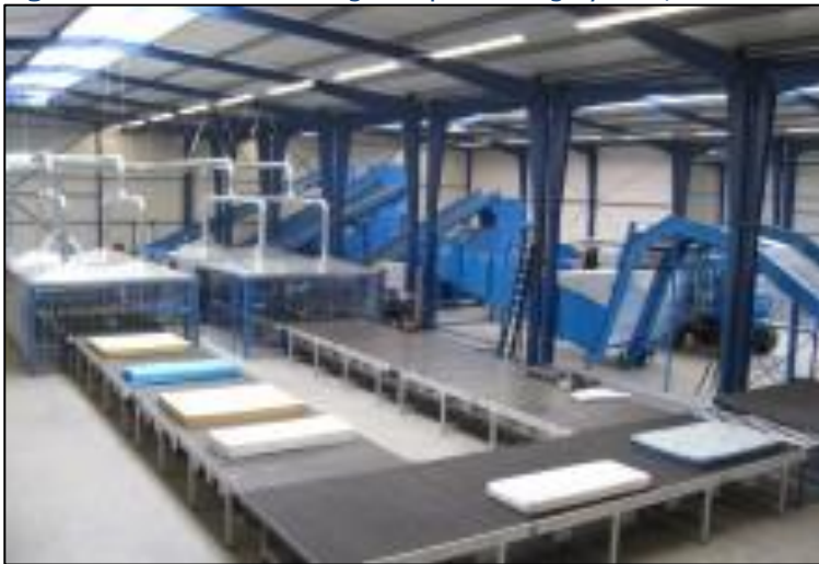
Figure 2.3 Mattress sorting and processing system, Retour Matras, Netherlands
